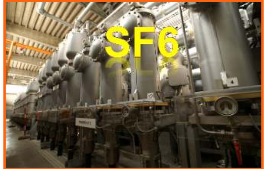
GIS: GAS ISSOLATED SWITCHGEAR
