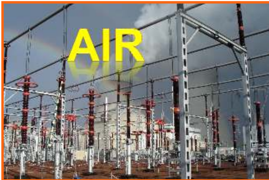
AIS: AIR ISSOLATED SWITCHGEAR
